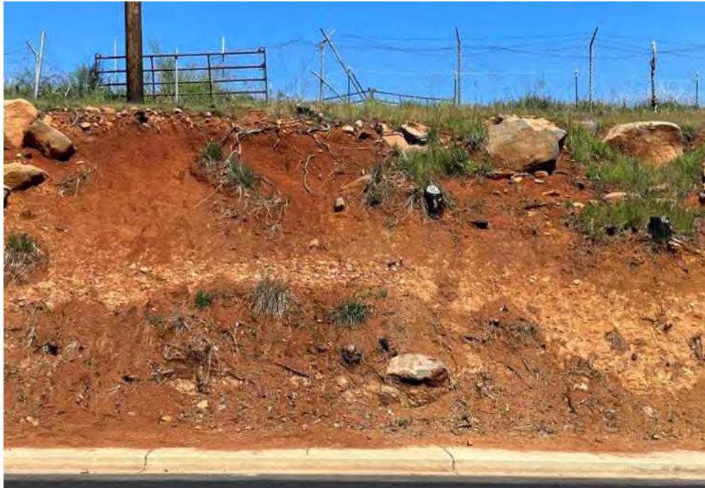
Photo 3: Gravelly volcanic mudflow bed below the basalt on Pearson Road. Note that erosion has removed most of the basalt at this location. Pearson Road.
