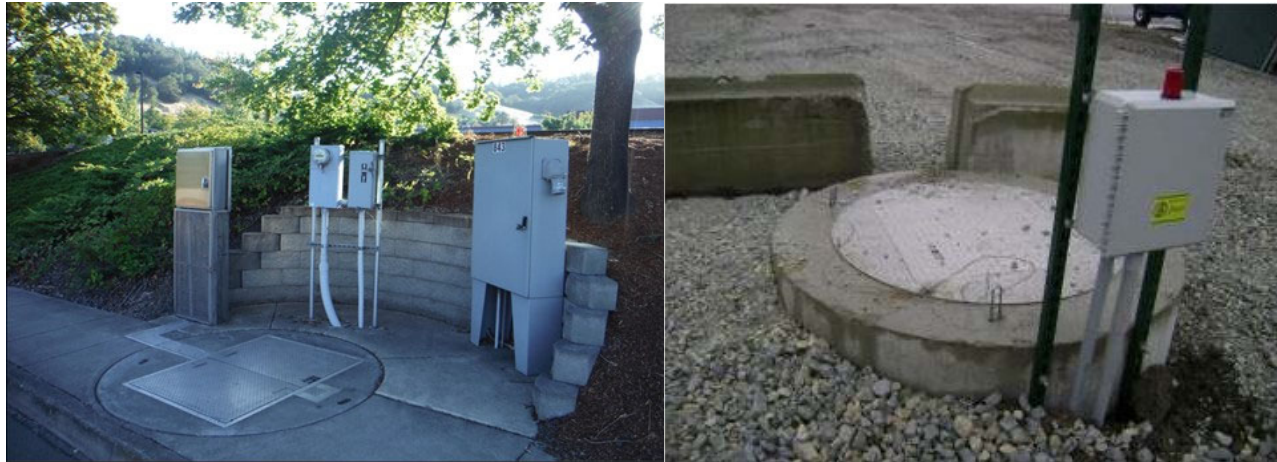
Figure 2-5. Examples of Below-grade Pump Stations (left: large, approximately 8 feet in diameter; right: small, approximately 3 feet in diameter)
