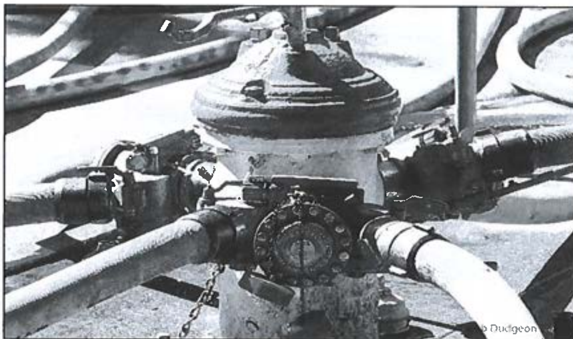
Figure 12 San Francisco AWSS hydrant direct connection of six attack hoses
