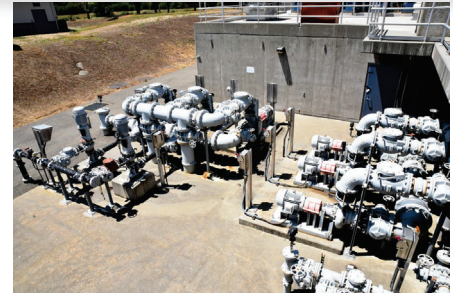
Influent, Recycle Pumps
