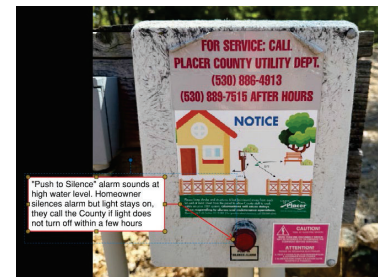
STEP monitoring station
