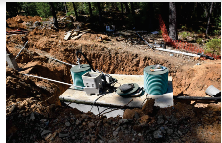
Septic Tank & STEP pipe
