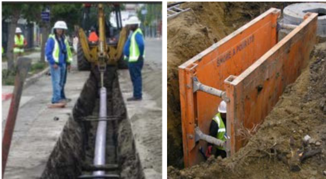
Figure 2-11. Typical Open-cut Pipe Installation (left: pipe layout; right: open cut and shoring)
