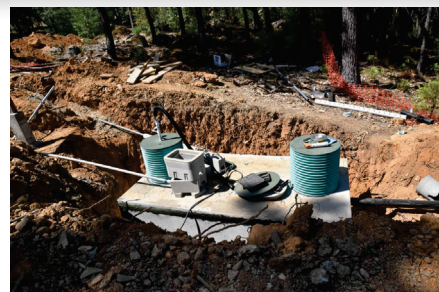
Septic Tank & STEP pipe
